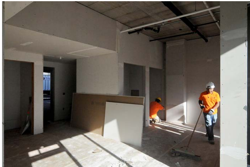
Crews with Columbia Drywall Systems work in one of the building's live/work units.
