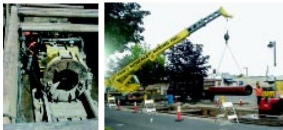
A pipe replacement project required tunnelling under the railroad crossing on Hall Boulevard.
